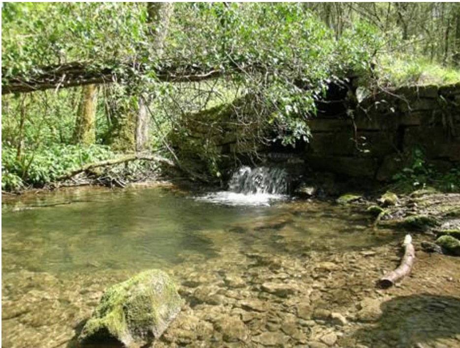
Figure 3.10 The culvert, tufa mound and scour pool on Slade Brook.
