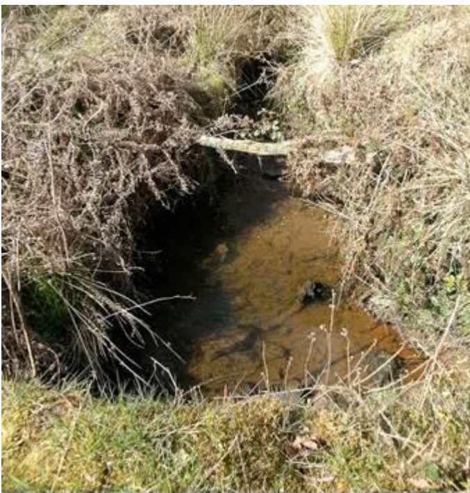
Figure 1.16 The main channel as it enters the culvert in the inclosure wall.
