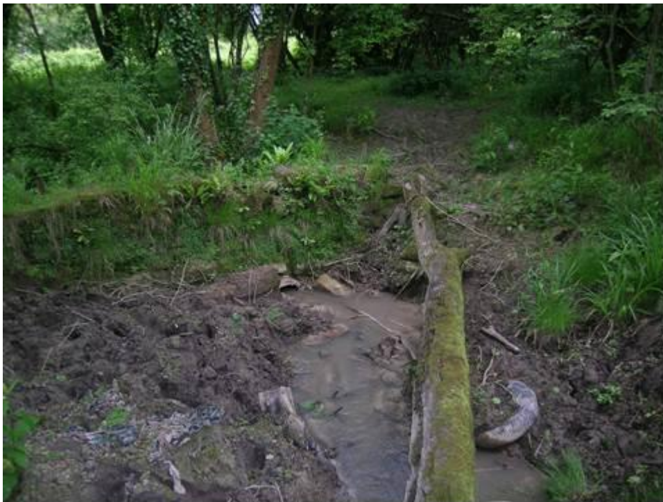
Figure 13. Stone wall built across the stream, and the small diameter pipe intended to take the streamflow.
