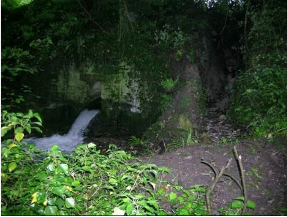
Figure 2.5 The impoundment at the top end of the walk, showing the breach.
