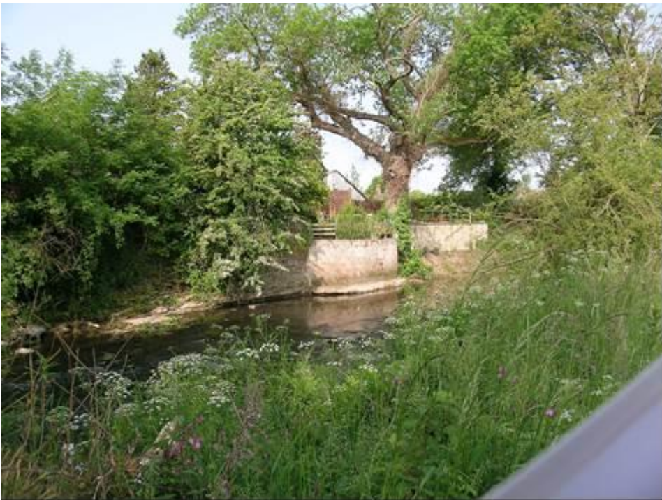
Figure 16. Concrete bank reinforcement adjacent to the cut-off meander (note the erosion visible under the toe of the reinforcement).
